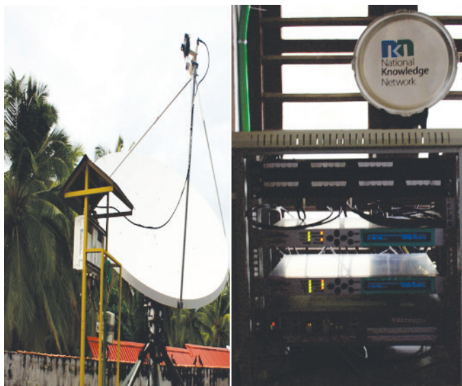
Fig 40 : High Capacity SCPC VSAT at Kavaratti, the U.T. of Lakshadweep Island for NKN Project
